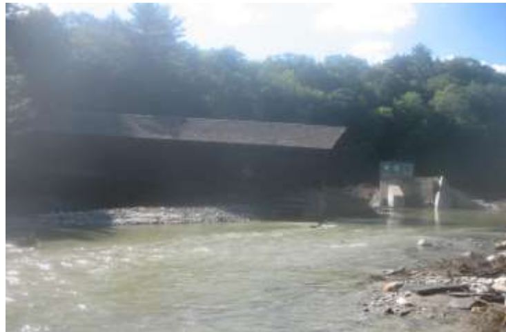
DAMAGE TO EUNICE WILLIAMS COVERED BRIDGE ON THE GREEN RIVER AT GREENFIELD, MA.
